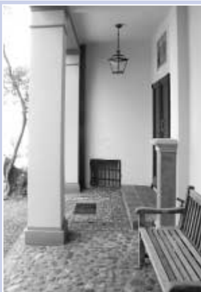
The pebble floor at the front door to the Papiniana was completely relaid.
