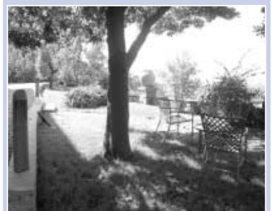
New grass was sown around the terrace and spectacular lookout point at the Papiniana. The area has now been well defined by a new retaining wall.
